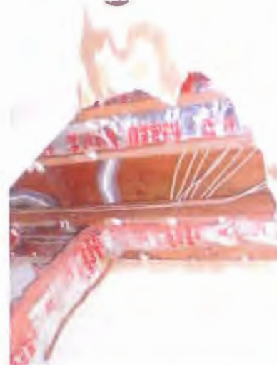
View of the ripped down bath ceiling.
