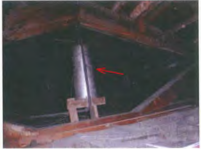
Attic still has the hot water heating system expansion tank in the attic.
