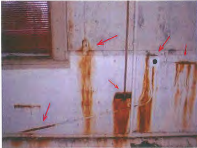
See water intrusion into the electrical boxes and raceways. This wiring needs replacement.
