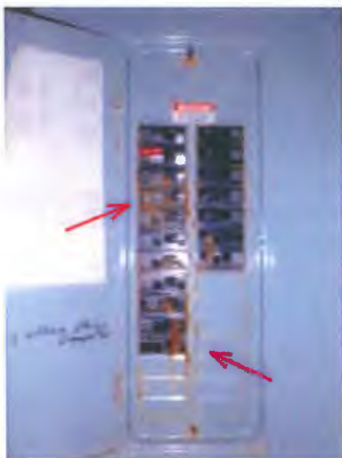
See rusting house panel. Panels were unsafe to open without service shut off.
