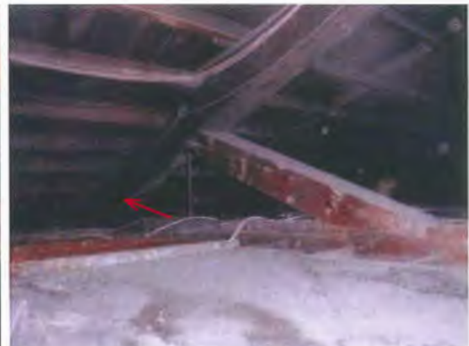
The ends of the heavy timber roof trusses are being wood rot damaged by the roof leaks.
