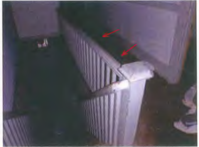
View down the stairs from the top floor. The stairwell railing is too short.
