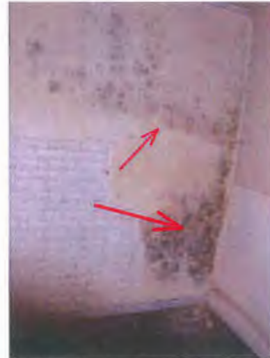
See mold developing around perimeter and especially at south side of the building.
