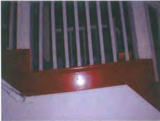
It's interesting that the stairs mid-run landing was intentionally installed out of level.
