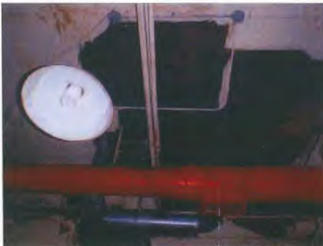
The roof leakage is destroying the building along the south side.
