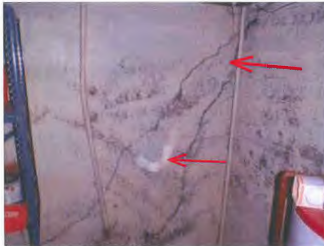
See basement SE area wall cracks.
