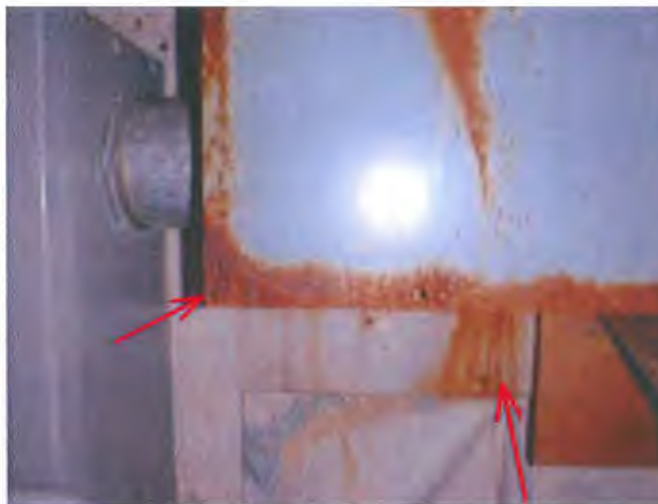
Rusted electrical service sub-panel wiring race-way.
