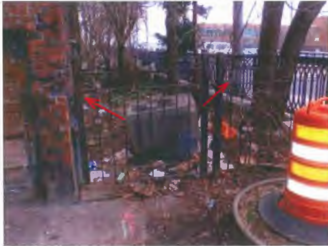
The rusting south side steel fencing needs repair and painting.
