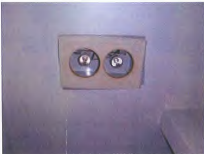
The once hot water heated building is now heated with lamps, baseboards and gas furnace.
