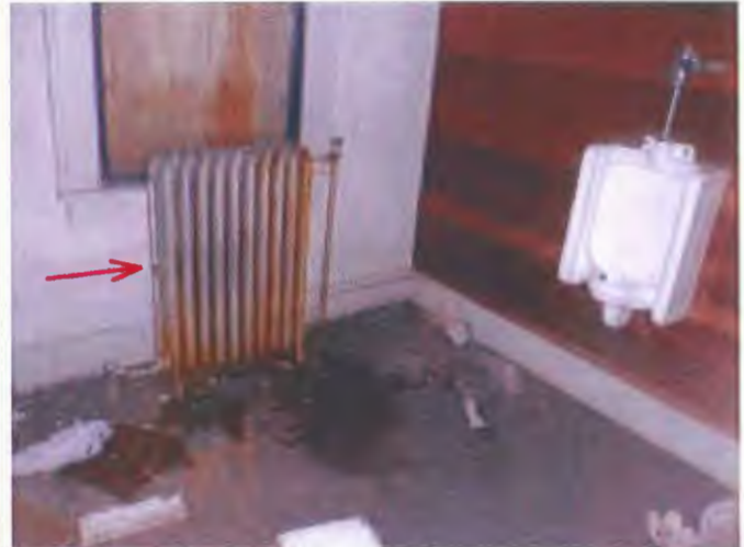
There are still some of the hot water heater radiators in the building.
