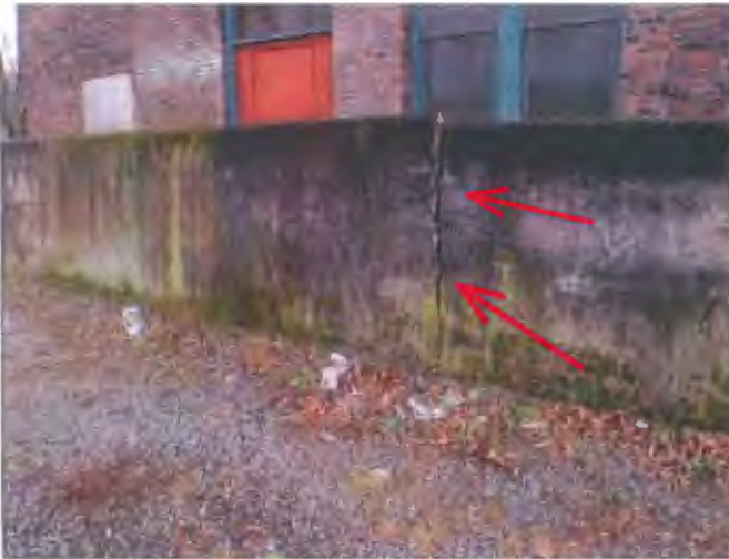
The newer north side concrete wall has cracked also. This may indicate more recent settlement.
