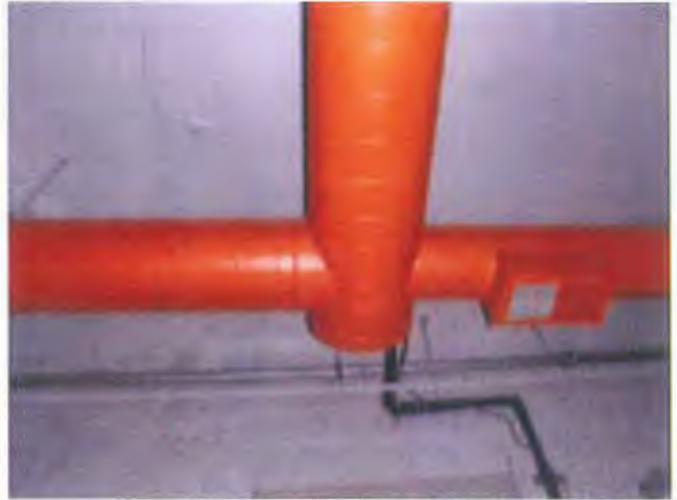
The furnace heat was distributed by these painted metal supply ducts.
