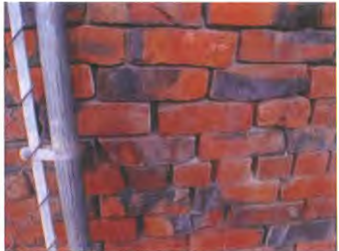
Close-up of the deep brick exterior mortar loss.
