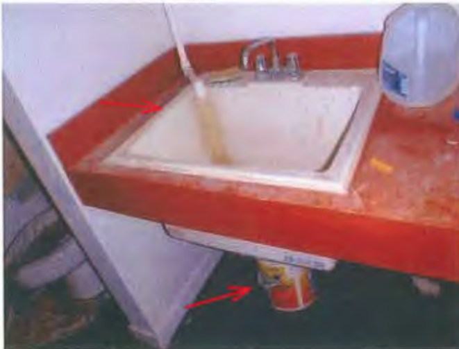
See stained sinks and buckets at the drain trap.
