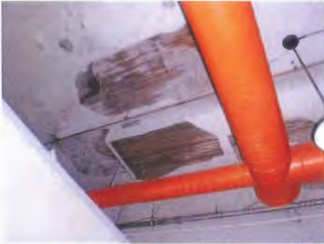
See roof leakage damage and mold in the first floor hall ceiling.
