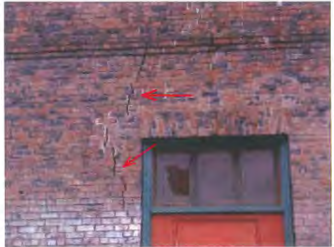
The crack runs the full height of the wall and indicates East end building settlement
