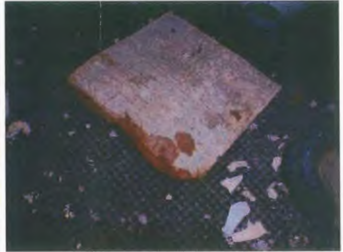
The ceiling tiles appear to be wood fiber but there appears to be an asbestos layer above them.
