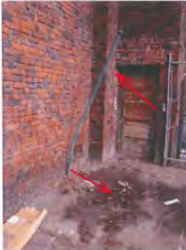
The SW corner of the property has an underground oil tank with bent vent pipes.
