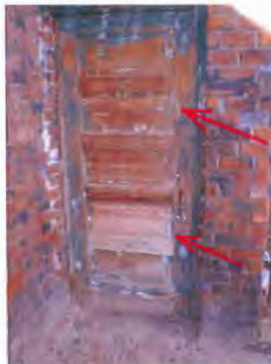
The SW corner external access door to a stairwell or old furnace flue chase was blocked.
