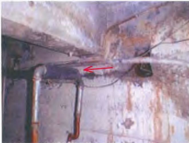
Auto radiator hose used to connect the water heater.
