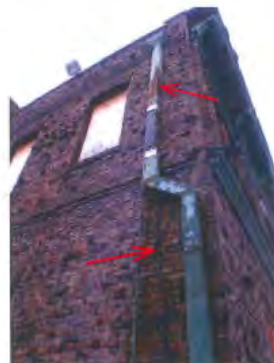
The metal NW building corner roof drain is also clogged and leaking.
