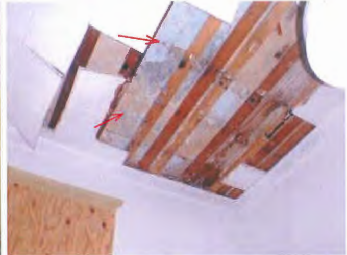
Here is a dryer area where that gray asbestos? fiberboard is visible above the ceiling tile layer.
