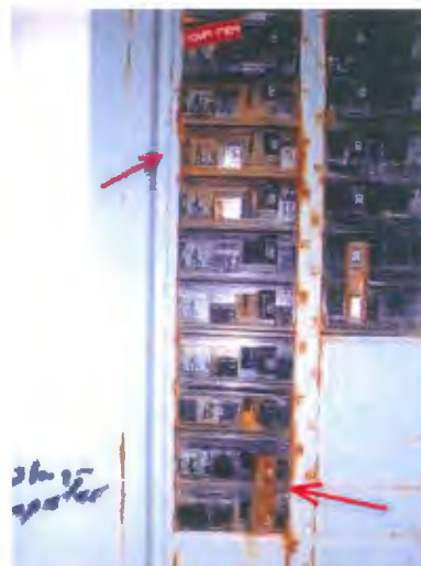
See heavily rusted circuit breakers and panel needing careful attention.
