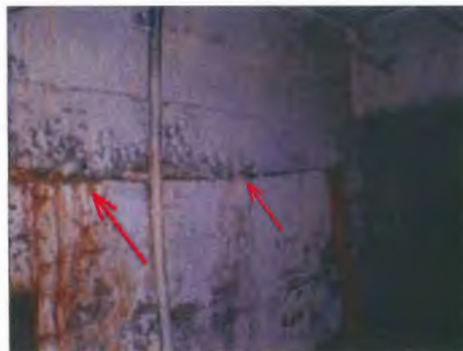
Water seeping in at the old basement concrete wall cold joints.
