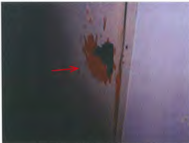
Any door locked was hacked until entry was gained. This is the basement stairs door.
