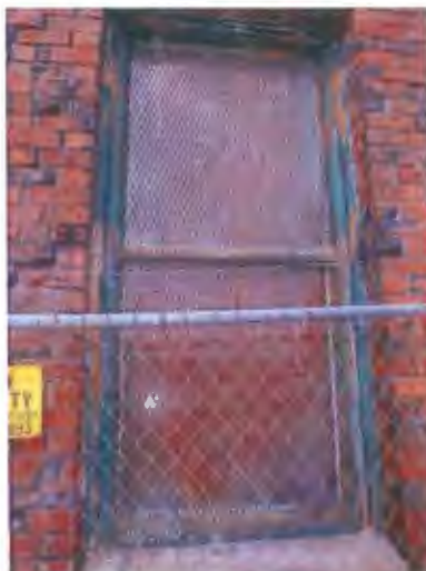
Some of old wood windows are still intact but need extensive restoration or full replacement.
