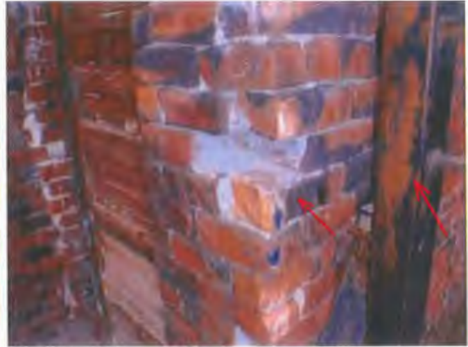
See the SW corner brick damage and rusting steel fence.
