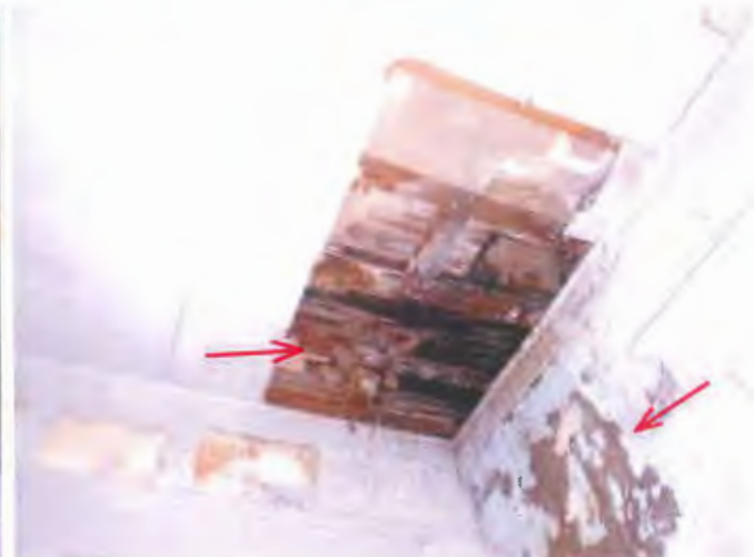
More roof leak ceiling and wall damage.
