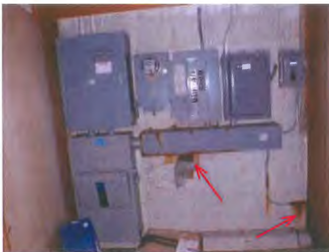
The NW main floor 400 AMP electrical service entrance panel with race-way and sub-panels.
