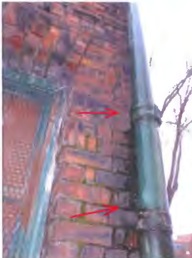
The SW cast iron roof drain is clogged and leaking down the building corner causing damage.
