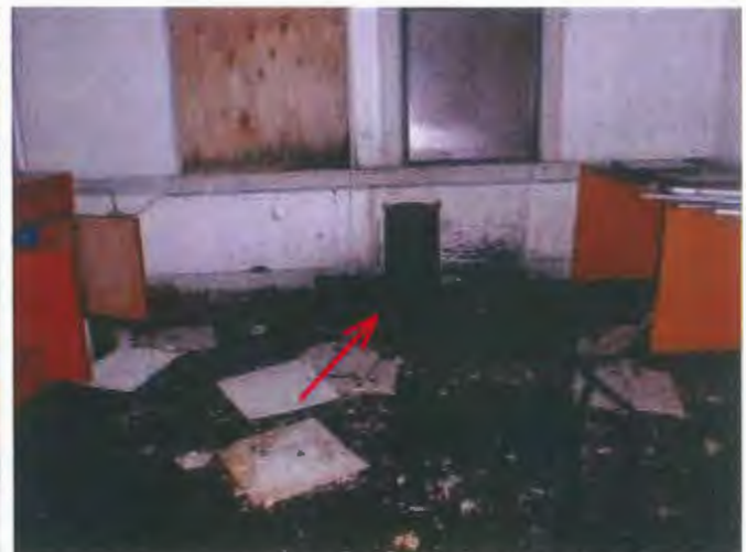
View of a wet moldy main floor south side office space.
