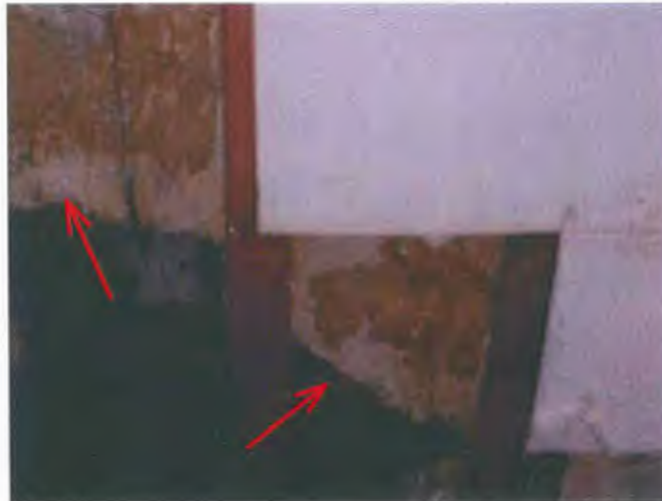
Hard to see in the dark wet building but this layer above the ceiling tiles may contain asbestos .
