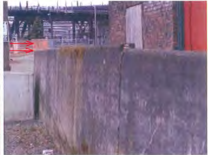
See the considerable site settlement at the northeast corner of the building and concrete wall.
