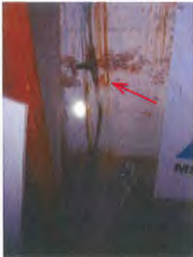
Basement south wall fuel oil supply lines. Probably there is an underground tank.
