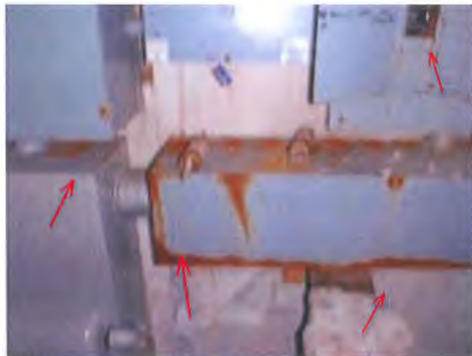
Water is damaging the electrical panels and they are becoming dangerous.
