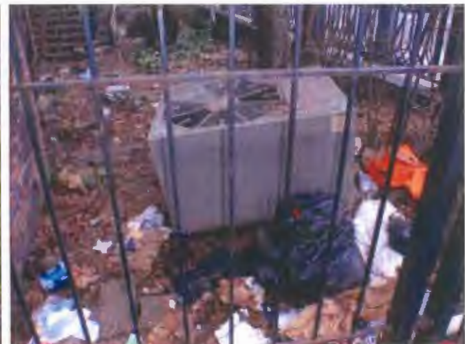
The south side AC compressor unit has been ripped off the building.
