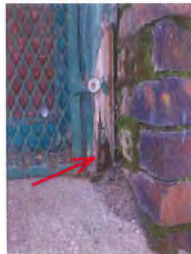
See the wood rot in the window trims and window jambs.
