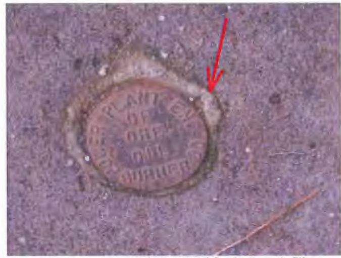
Southwest corner underground fuel oil tank fill cap. Tank needs decommissioning?
