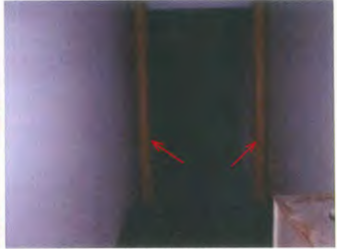
The roof structure is wood timber trusses with steel columns and beams for second floor support.
