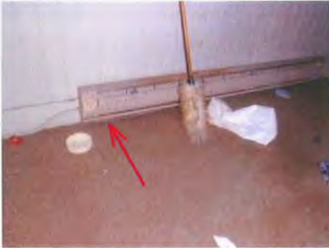
Most of the second floor is heated or has back-up electric baseboard heaters.
