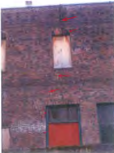
Serious north brick wall settlement crack. The south wall is cracked too.
