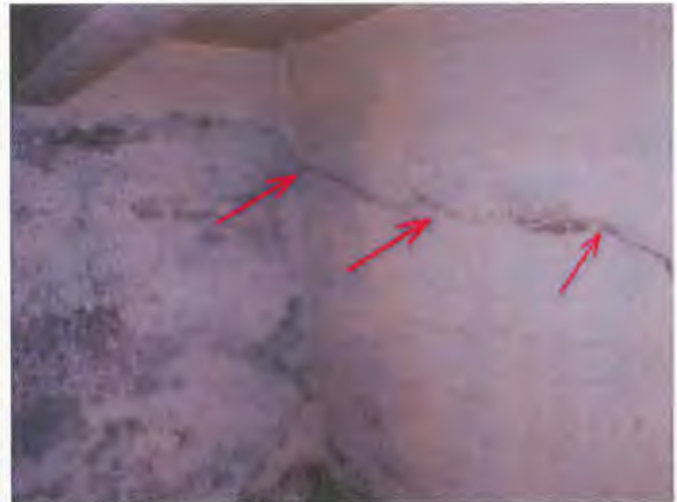
Some basement wall cracking appears to follow old concrete placement cold joints.
