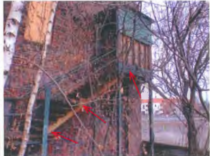
The external stairs need safety modifications. Trees need to be cut back off the building.
