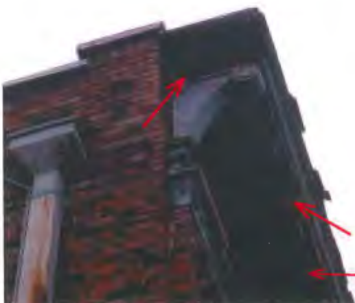
The front corbelled soffit has extensive wood rot damage.
