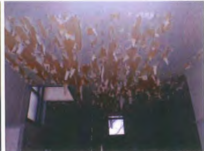
See damaged east main floor room's ceiling. A lead paint nightmare?
