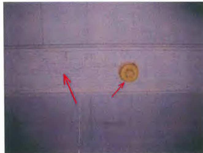
Lots of peeling lead paint and of course the old smoke alarms need replacement.
