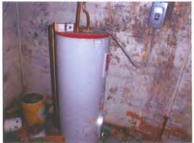
The electric water heater in the basement near the old boiler. Needs seismic strapping installed.
