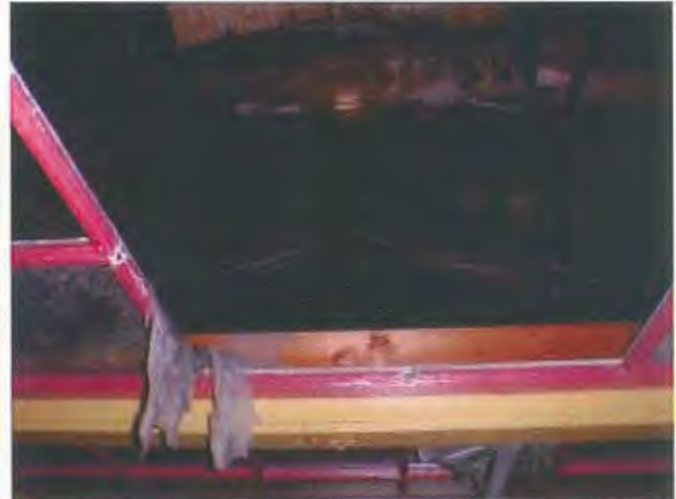
See the wet roof sheathing and solid wood timber trusses of the roof structure.
