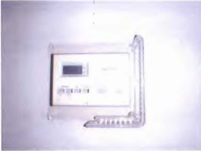
The furnace thermostat still remains intact.
