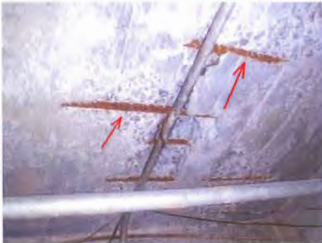
See the rusting exposed rebar in the basement ceiling below where the fire truck was parked.
