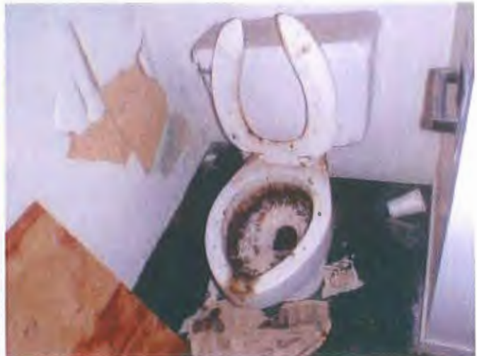
The plumbing has been abused and will need full flushing of all drains and extensive restoration.
