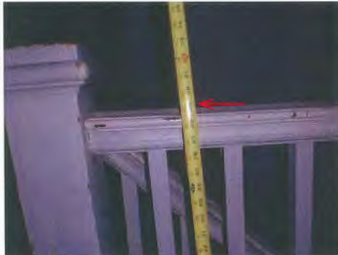
Stairwell railings are only 29" tall. Need 36" Min. but commercial usually 42" for fall safety.
