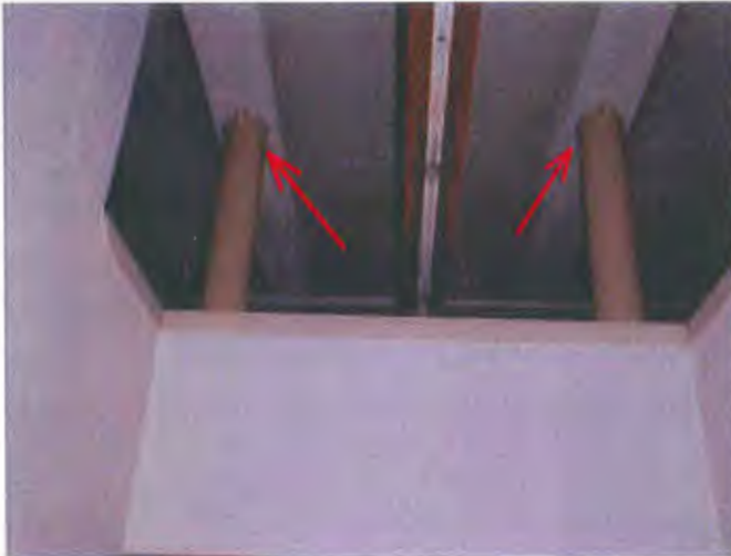
See tops of the steel columns supporting beams supporting the top floor wood joist system.
