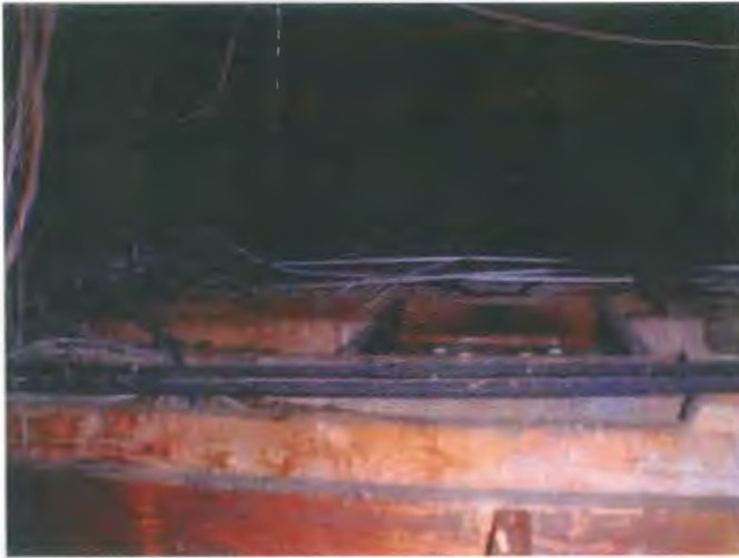
The building has no attic insulation.
