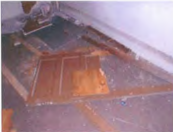
Many interior doors are now just broken scraps.
