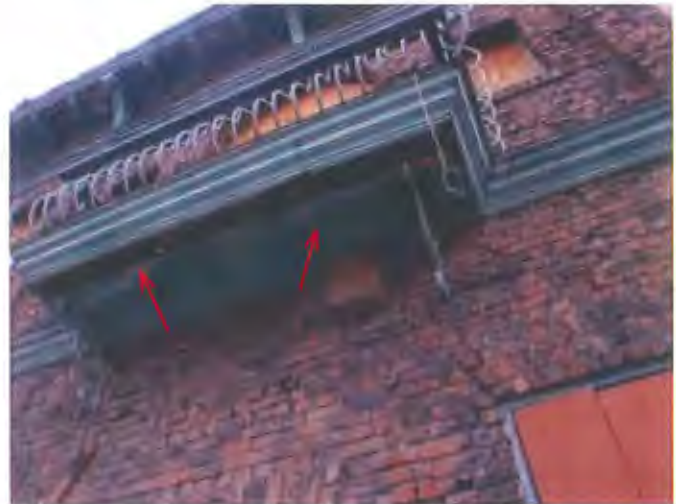
Water induced wood rot in the front balcony.
