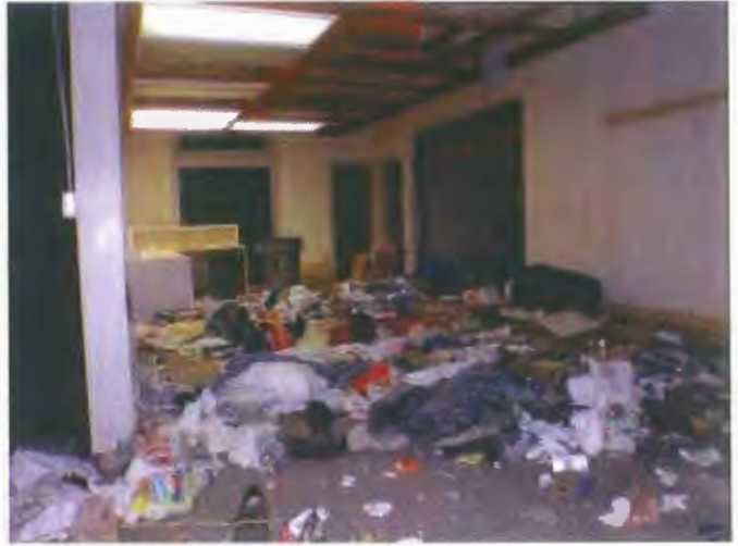
The upstairs needs considerable clean up and trash removal.
