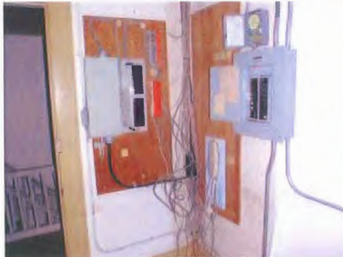
It's amazing that the building's copper wiring hasn't been stolen.
