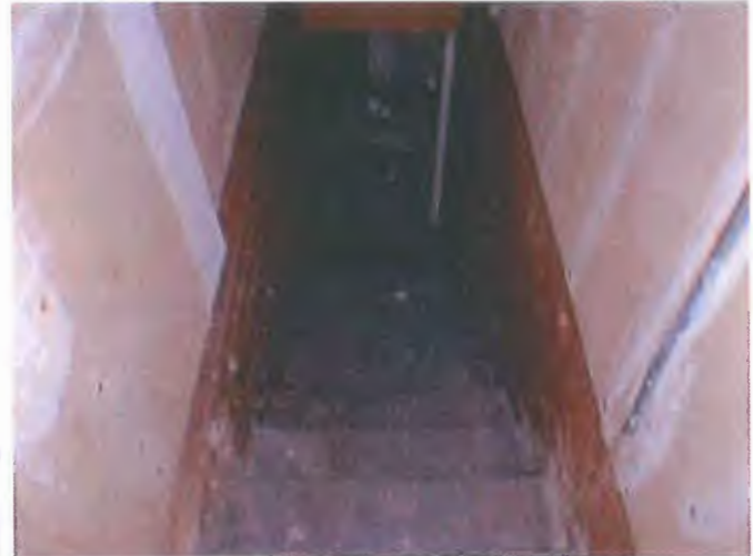
Now down to the partial basement. The basement concrete stairs need a handrail installed.
