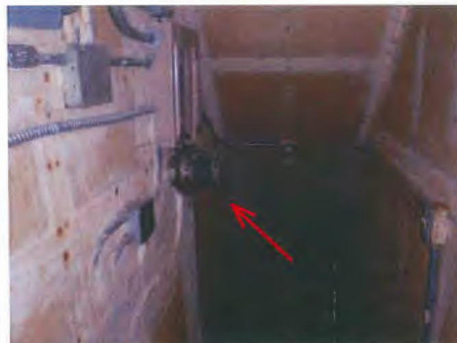
This panel and meter protrude into the basement stairwell and maybe should be moved.
