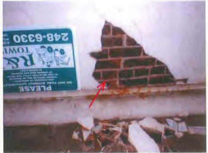
The building's exterior walls appear to be full brick and will need serious seismic upgrades.
