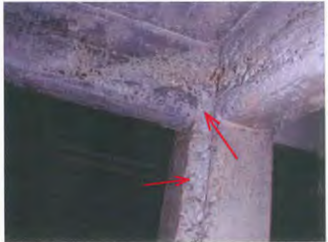
Rustic spawling basement column and floor beam concrete.
