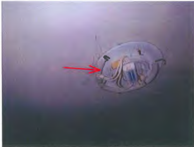
Lots of damaged light fixtures.
