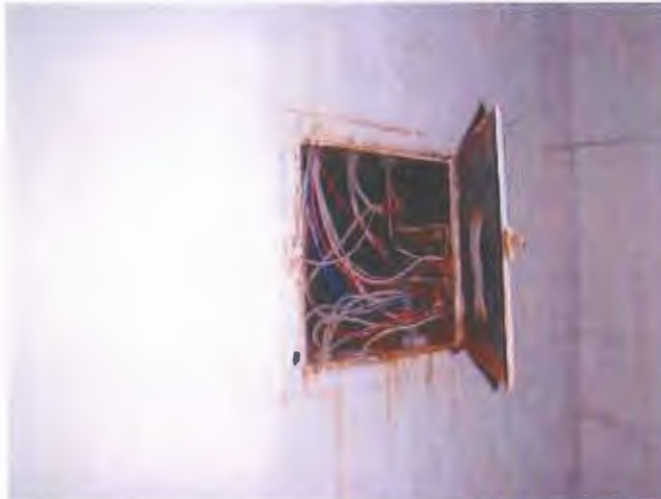
Rusting converted fuse panel now wiring splice panel. The roof leaks are destroying the building.
