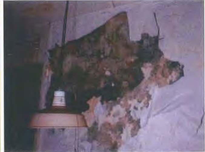
See the multi-colored molds growing in the wet south walls.
