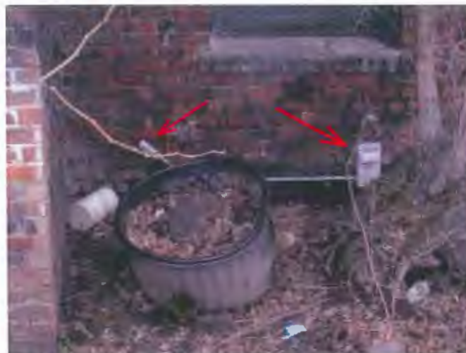
The south side air conditioning wiring has been damaged.
