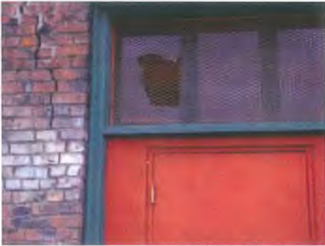
Lots of broken and boarded up windows.
