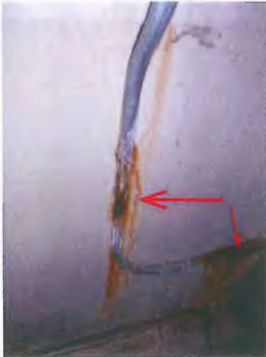
See seriously corroded electrical conduit too.
