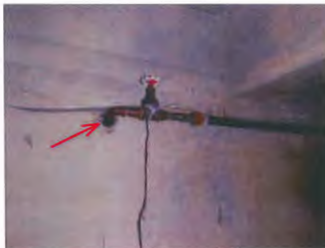
Building appears to have a newer copper water service line installed through west basement wall.
