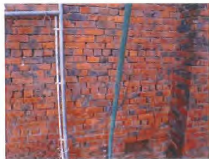
Extensive brick exterior mortar loss. The brick building's exterior needs full refurbishing.
