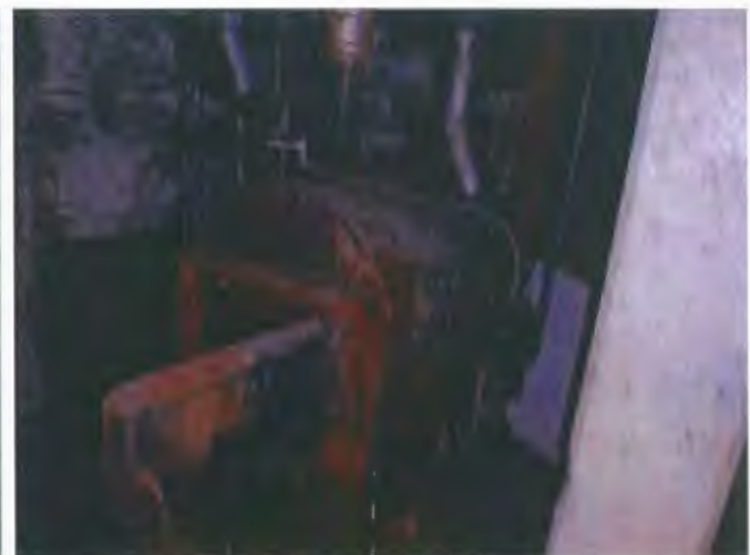
The old abandoned oil fired hot water heat 'boiler' in the south end of the partial basement.
