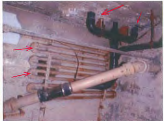
NW basement corner had hot water heat below the main floor baths to prevent pipes freezing.
