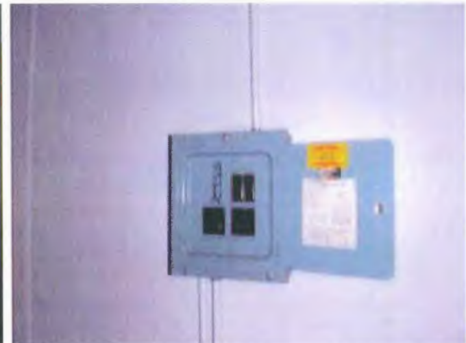
The building does have areas yet undamaged by the roof leaks and intact electrical sub-panels.
