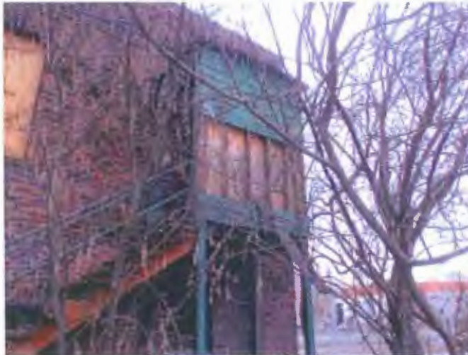
The trees need to be pruned back off the building.
