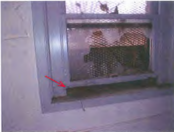
Need open broken windows boarded up to keep rodents out.
