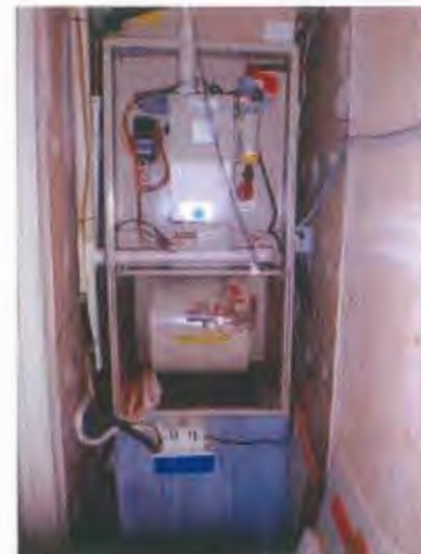
The Lennox 90+ gas furnace located in the basement stairwell.
