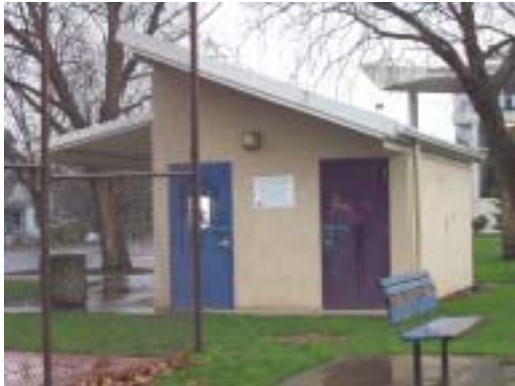
Restroom conditions have deteriorated.
