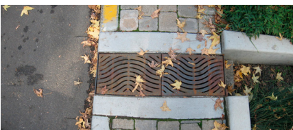
Stormwater Planter inlet (Urban Accessories' Wave Trench Grate)
