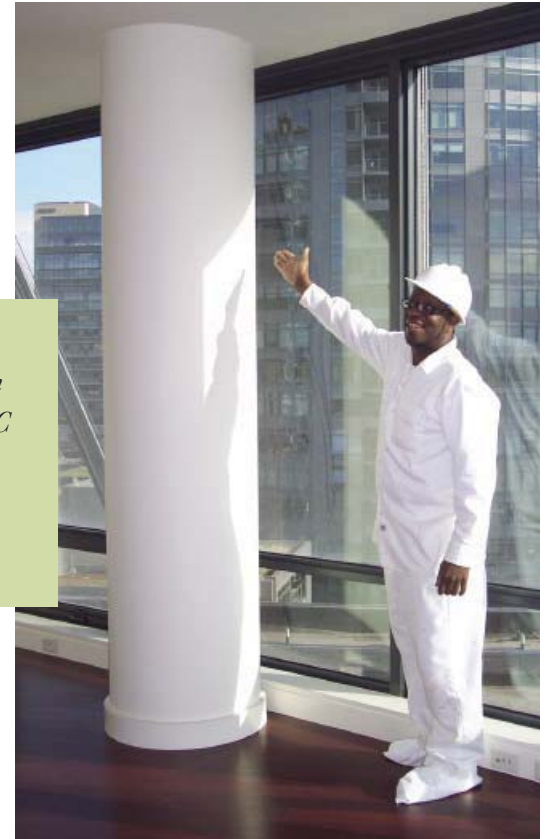
Nathaniel Hartley displays the high quality, smooth plaster he skillfully applied to a cement pillar in the Ardea Apartments in the South Waterfront.
