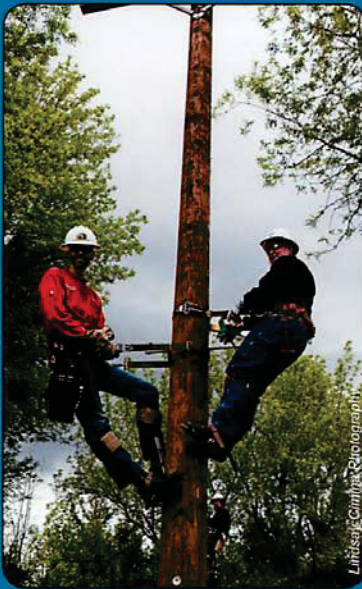
A Careers for Women Day attendee learns to climb a utility pole in Portland General Electric's workshop
